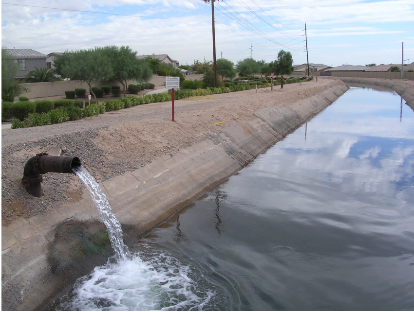
Extraction well 33A system discharge into the Roosevelt Irrigation Canal (RID)
