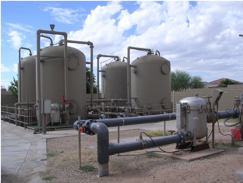
This is the extraction well 33A treatment system for TCE treatment. The system is designed to extract contaminated groundwater from Subunit A at the northwest portion of the plume and treat it for TCE prior to discharge to the Roosevelt Irrigation District (RID) Canal. The system located in the front of the picture is actually part of a sand trap pre-filter that filters the water before it goes to the carbon vessels.
