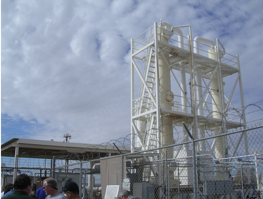
This is the Main Treatment System located at the PGA-North (Unidynamics) site. The system treats contaminated groundwater for TCE and perchlorate at the main site, and then the water is reinjected into the aquifer through a network of injection wells in Subunit A.
