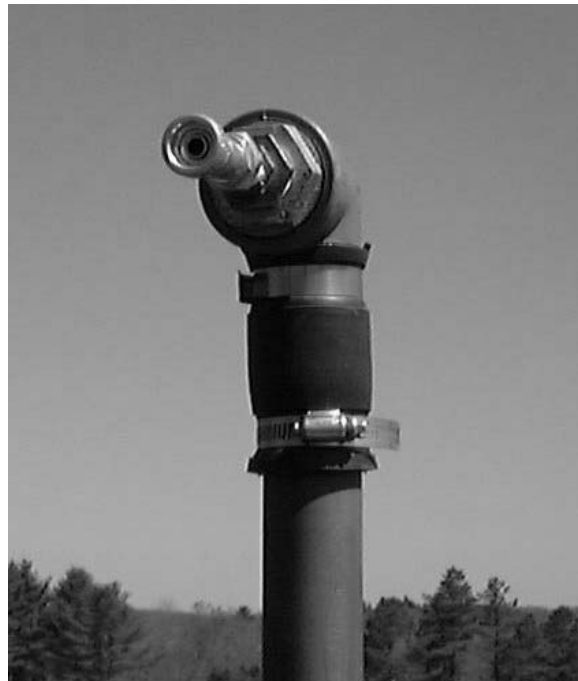
Figure 7.13 Close-up of quick-connect at top of 3.2 cm i.d., sch-80 PVC pipe to prevent gas pressure release at shut-in
