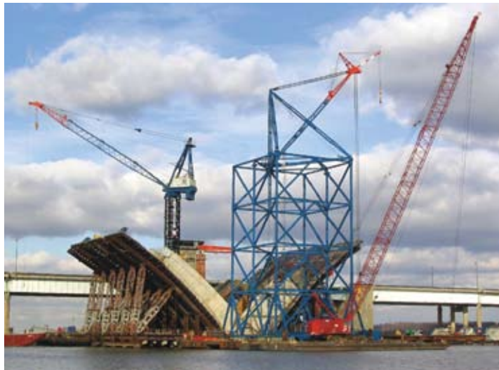
In 2004, the team working on the Woodrow Wilson Bridge Project in the Washington, DC, metropolitan area (shown here during construction) conducted a formal risk management assessment for the entire project. The following were among the critical program elements identified for risk assessment: project-wide security, fabrication and availability of materials, incident management, project schedule, environmental commitments, utility construction conflicts and delays, design management review and oversight, change orders, maintenance of traffic, and work zone safety. Photo: Woodrow Wilson Bridge Project
