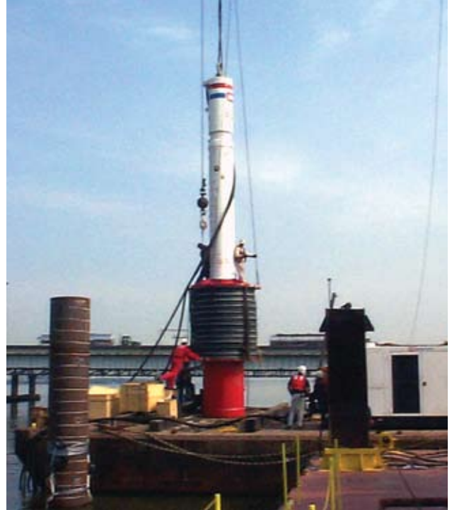
Geotechnical applications in the field. Workers are driving open-end piles with a double-acting hydraulic hammer on the new Woodrow Wilson Bridge near Washington, DC. Photo: Jerry DiMaggio, FHWA
