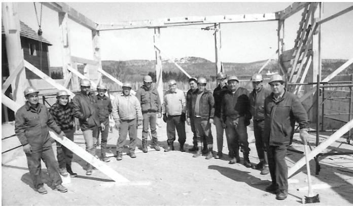
Great Hall construction crew 1971 (L to R): Norman Deschampe, Sr., Ernest Spry, Gordon LeGarde, Fred “Bud” Haylock, Raymond Duhaime, Theodore Kozlowski, Skipper Roberson, Herman Hendrickson, Kenneth Sherer, Larry Dahl, Steven Hunter, Anthony LeSage, Roger Deschampe
