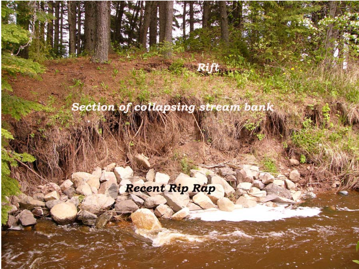
Figure 12. This east view shows a collapsing section of stream bank, recently riprapped, just below the old ford on the east side of Grand Portage Creek (Digital photo by the author, 6 June 2005).
