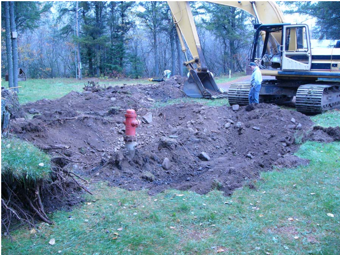
Figure 7. This northwest view shows hydrant replacement work in the parking lot clearing south of the Maintenance Shop in October 2004. The backhoe excavations, monitored by NPS management staff, uncovered a mix of apparent late-nineteenth century household debris in previously disturbed soil contexts. Among the observed materials were pieces of spiral-fractured, mammalian bone, machine-cut and wire nails, stoneware crockery (including some RED WING), transfer-print ceramics, brown bottle glass, and other materials. (Digital photo by the author, 20 October 2004).
