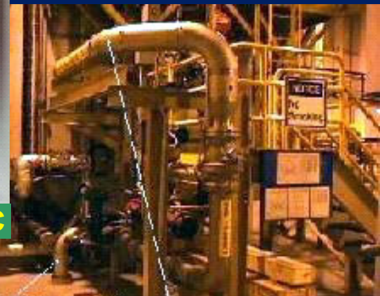
LFG-fired Boiler Ft. Wayne, IN
