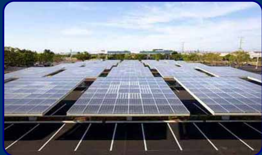
Photovoltaics Produce Electricity Covered Employee Parking
