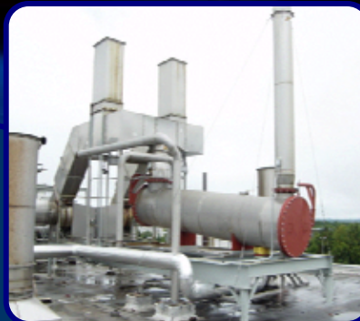
PC Stack Heat Recovery
