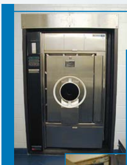
Autoclave The facility's autoclave is a unique piece of equipment because it accepts contaminated instruments on the BSL3 suite side, sterilizes the instruments with pressurized steam, and allows extraction of sterilized instruments outside the suite. A rubber bioseal around the Autoclave helps assure containment of BSL3 agents within the Biocontainment Suite.
