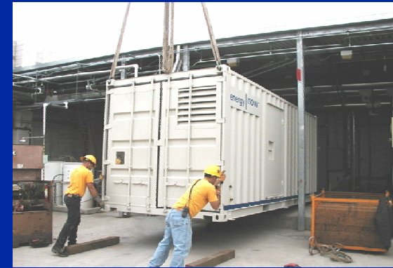
375 kW Cogeneration unit in Pleasanton, CA
