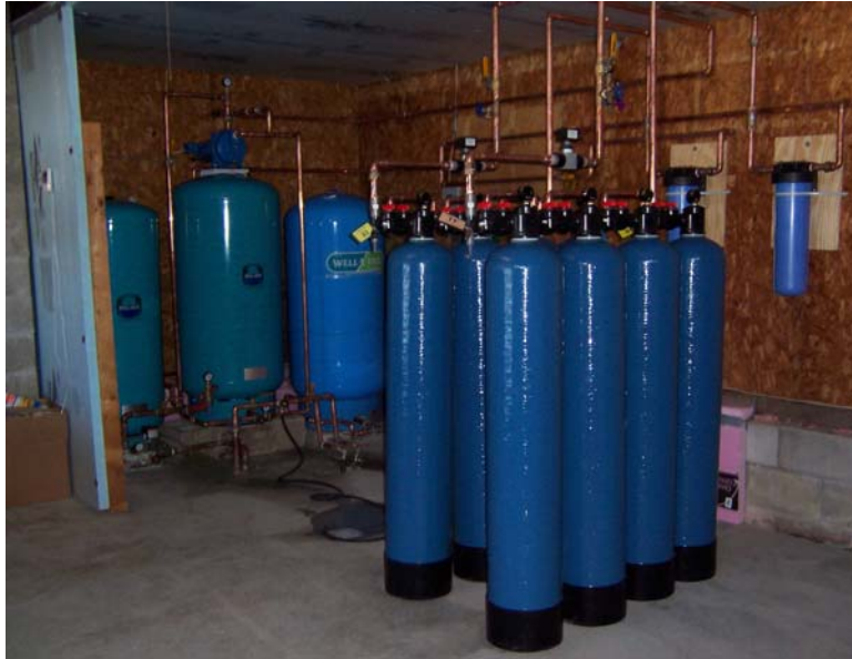
Figure 4-5. As/1400CS Arsenic Adsorption System with Adsorption and Oxidization Columns Shown in Foreground, 25- \mu m Sediment Filters Attached to Wall, and Hydropneumatic Tanks in Background
