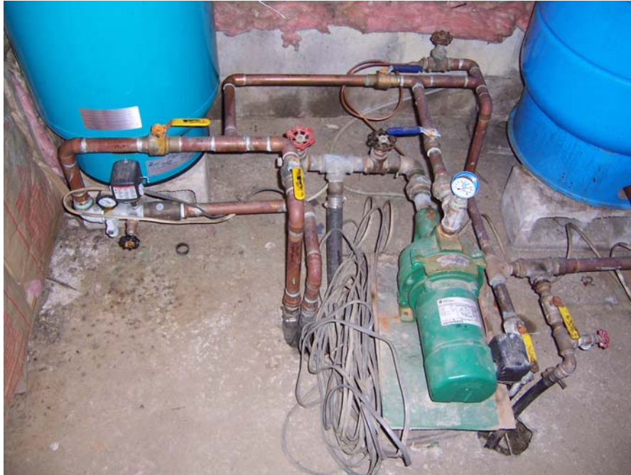
Figure 4-2. Pre-Existing Water Supply Pump, System Piping, and Hydropneumatic Tanks (shown in the background)
