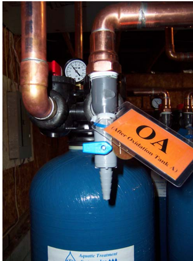
Figure 4-6. Close-Up View of a Sample Tap (OA), a Pressure Gauge, and Copper Piping at Head of a Column
