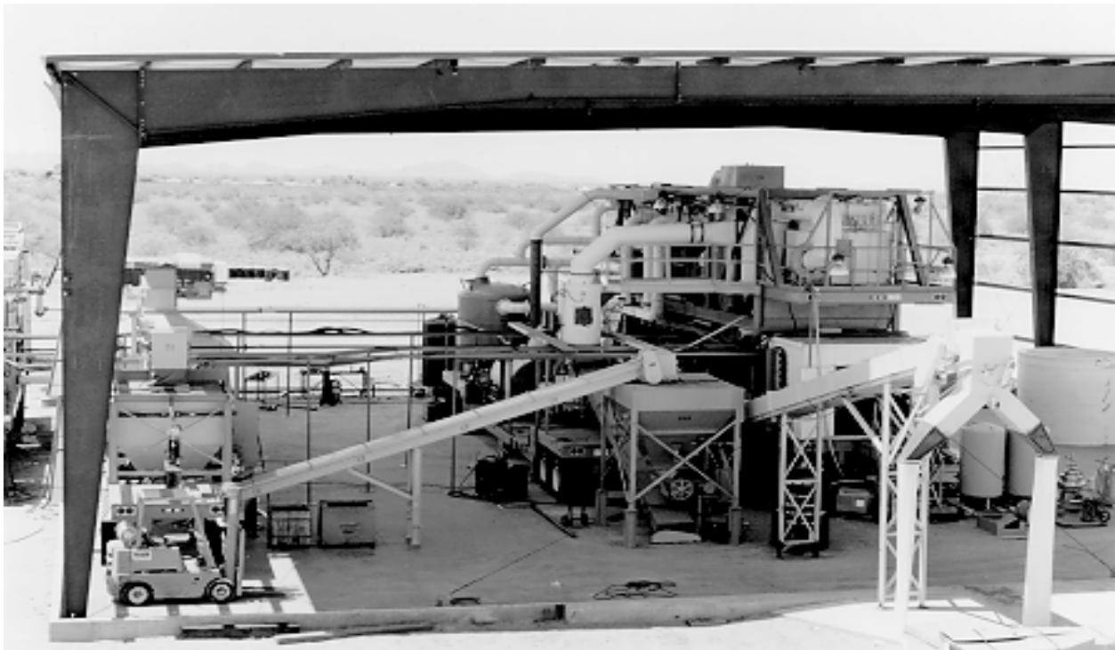
Desorption and Vapor Extraction System (DAVES)
