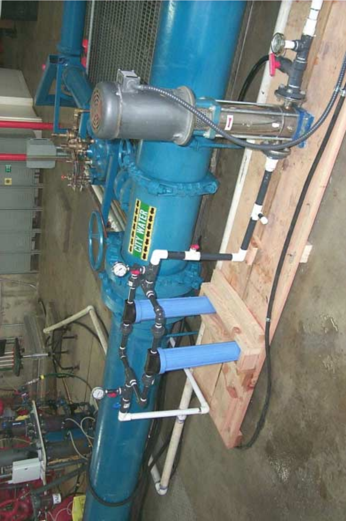
Photograph 2: Membrane Element Module Test Unit showing prefilter housing and high pressure pump
