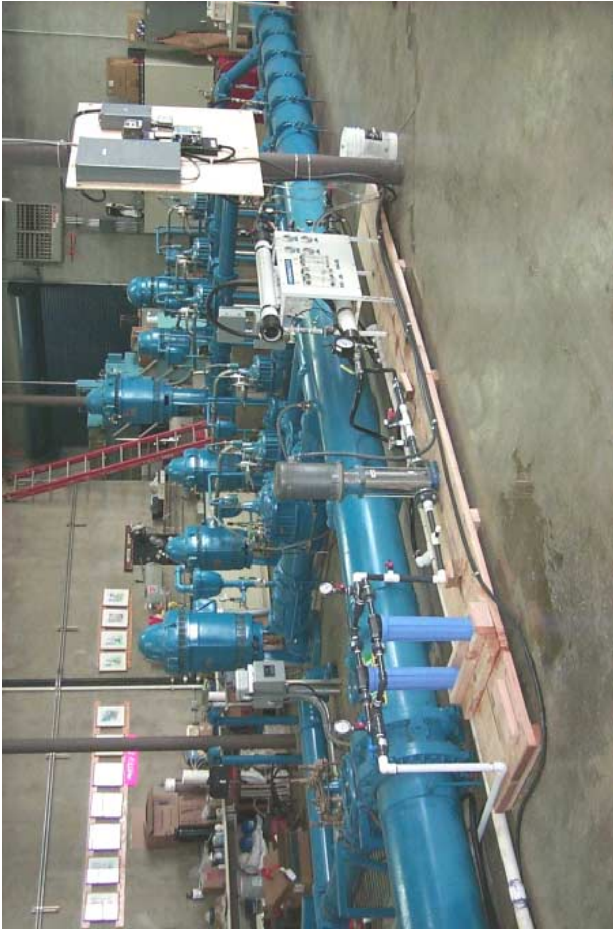
Photograph 1: Membrane Element Module Test Unit showing prefilter housing and high pressure pump
