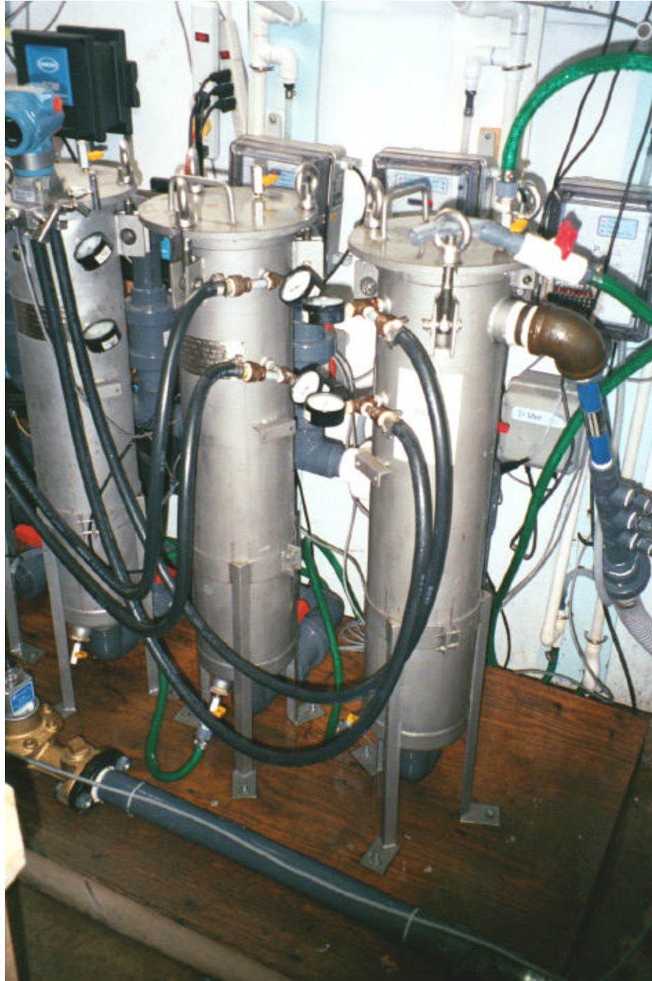
Photograph 21. Treatment System as Installed at Burnside Borough (including pressure vessels, pressure gauges and particle counters)
