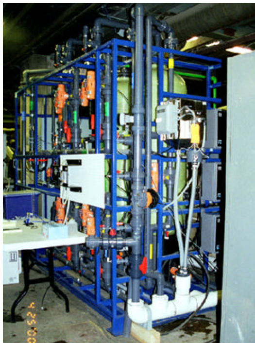
Photo 2. Side view of the Kinetico SW224 Filter System at the University of Minnesota.
