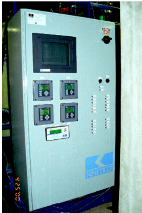
Photo 1. Front view of the was Kinetico SW224 Filter System at the University of Minnesota
