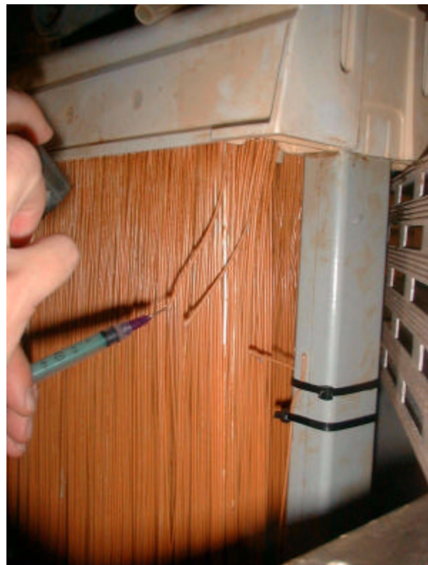
Figure 4-17. Seal Repair of Damaged Fiber with Epoxy
