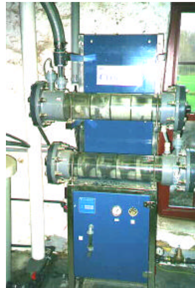
Photograph 2.3 Sodium Hypochlorite Generator
