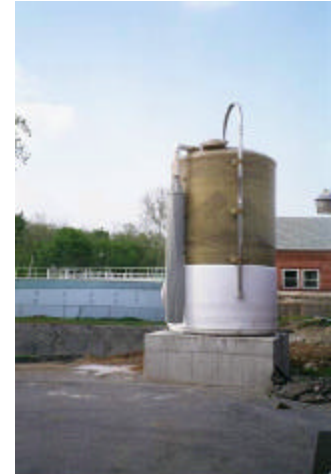
Photograph 2.1 Brine Bulk Saturator Tank
