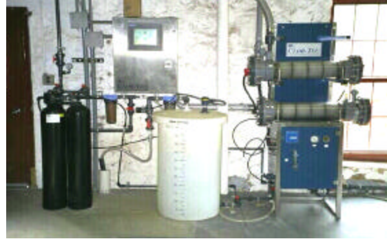
Photograph 2.2 Softener, PLC, Brine Day Tank and Hypochlorite Generator
