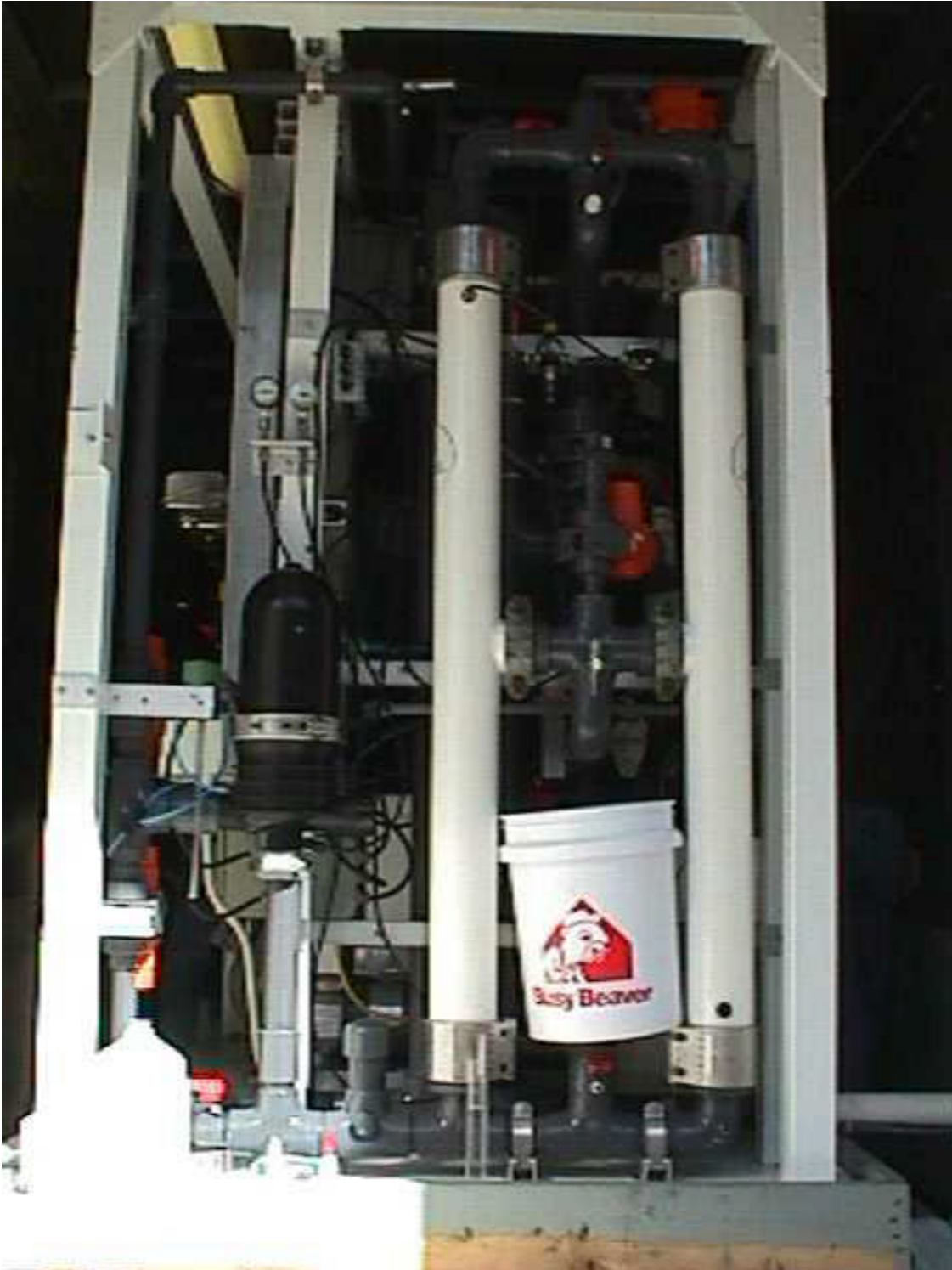
Photograph 1. Aquasource Ultrafiltration System Model A35 showing piping, membrane modules and prefilter.
