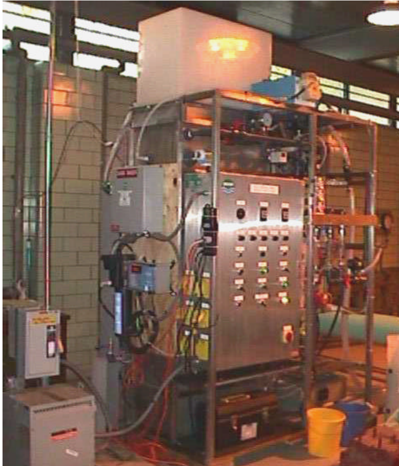
Photograph 1. The ZENON Environmental Inc. ZeeWeed® ZW-500 UF Drinking Water System showing control panel, process tank, bleed pump and ancillary equipment.
