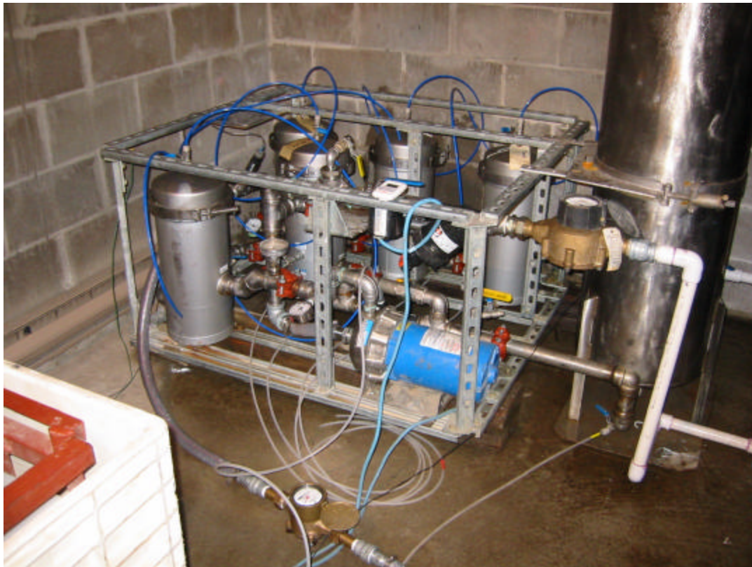
Figure 2-3: Close-up Photo of CampWater System.
