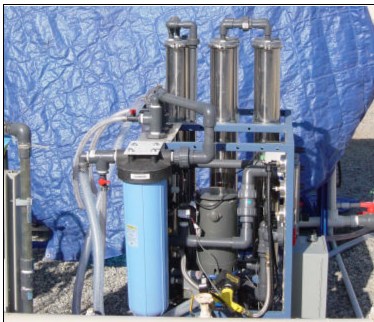
Photograph 3: Pre-Filter to Watts Premier M-15,000 RO Treatment System
