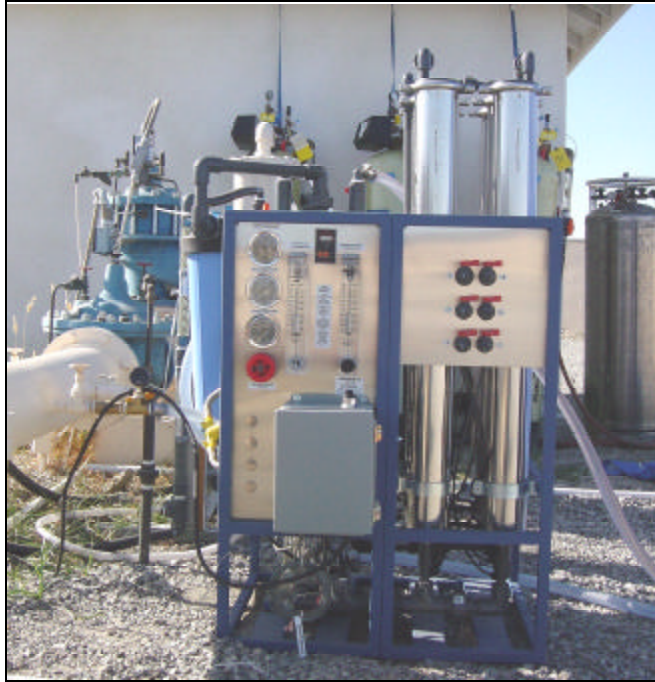
Photograph 2: Watts Premier M-15,000 RO Treatment System at CVWD Well 7802
