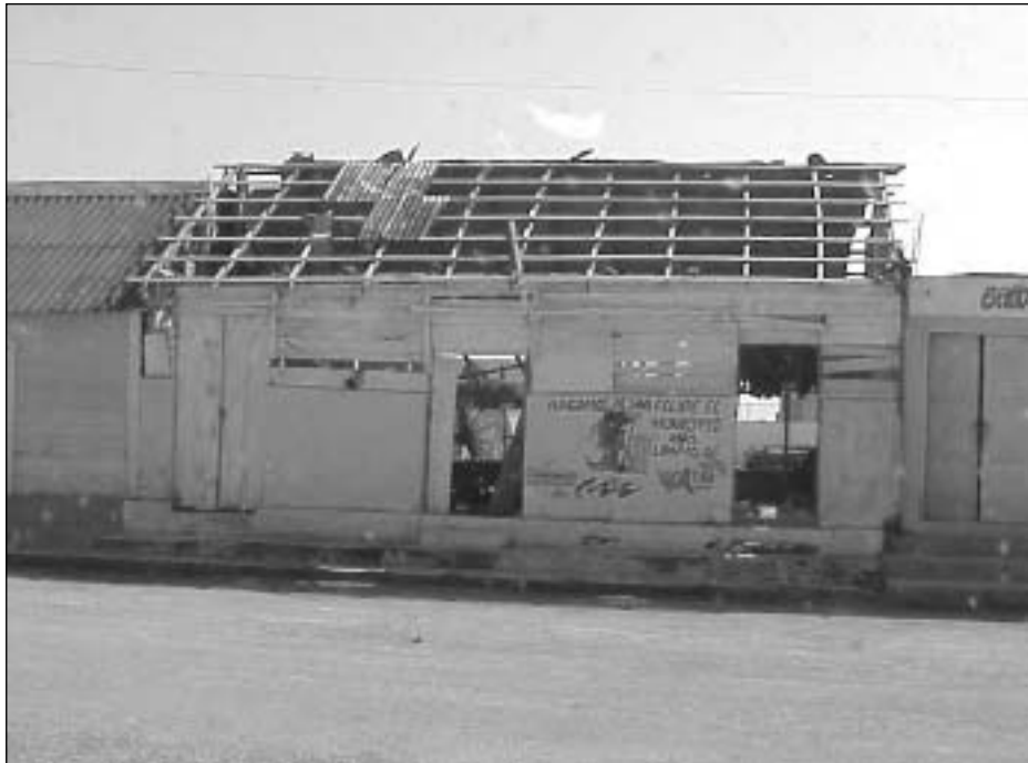
Roof blown off building damaged by Hurricane Isidore in September 2002 (photo by USAID/OFDA).
