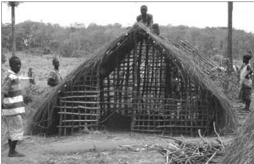
Men thatching roof of new IDP shelter, Maimu III (photo by Fiona Shanks, USAID/OFDA).
