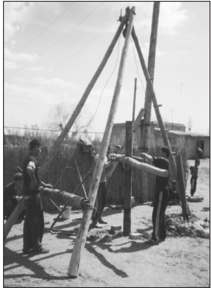
USAID/OFDA funded the construction of neighborhood wells to assist the drought-stricken residents of Khalkabad, Uzbekistan (photo by Gilbert Collins, USAID/OFDA).
