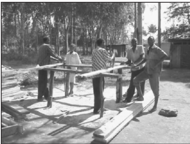
Local IMC staff begin construction of a new therapeutic feeding center funded by USAID/OFDA in Gasorwe, Muyinga Province, Burundi (photo by Pia Wanek, USAID/OFDA).
