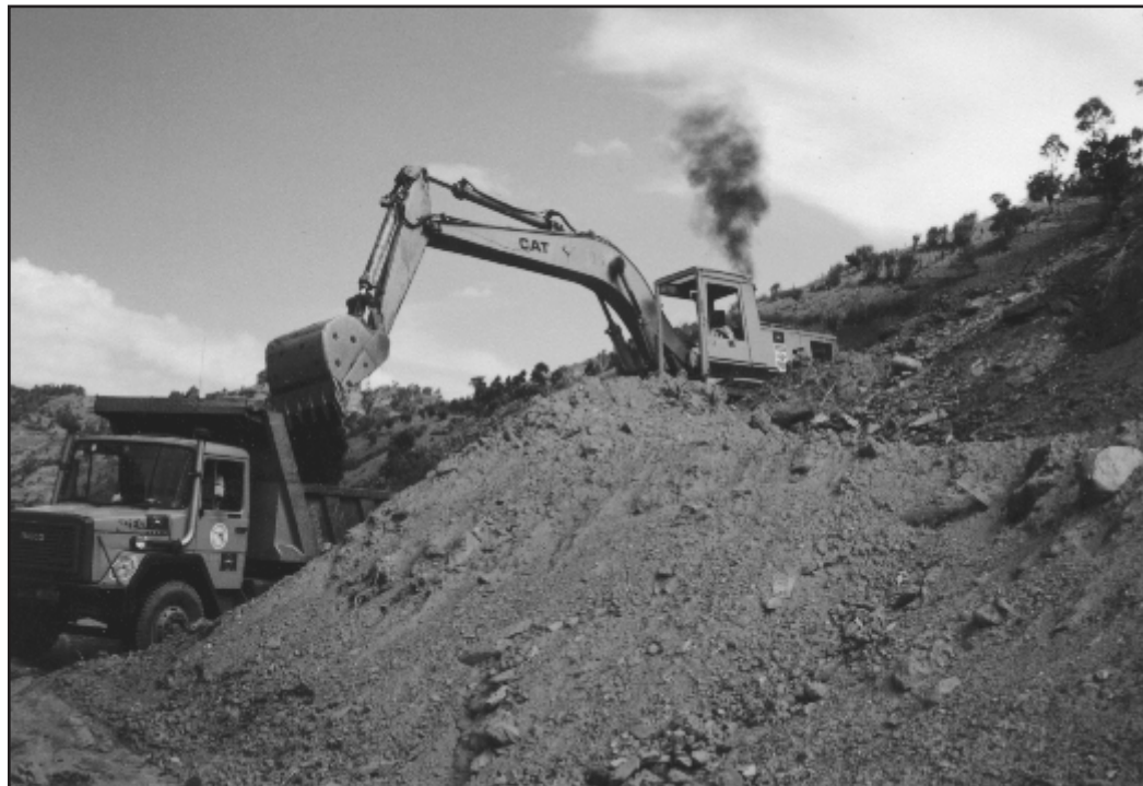
As part of a USAID/OFDA-funded seed multiplication project, German Agro Action (GAA) is reconstructing roads in North Kivu to facilitate trade in the region (photo by Tim McRae, USAID/OFDA).
