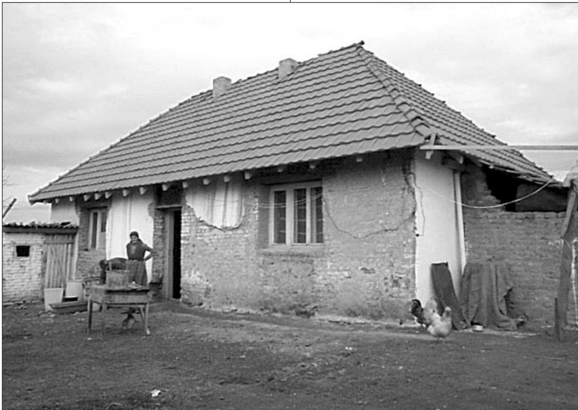
A USAID/OFDA-funded roof repair is completed in Kosovo (photo by Paul Majorowitz, USAID/OFDA).
