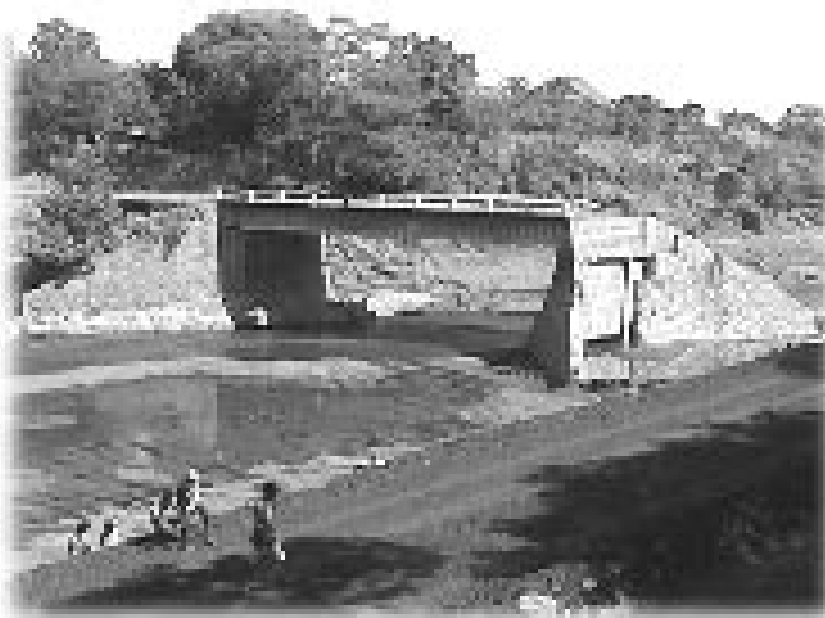
A damaged bridge north of León along the Chiquito River isolates local residents (photo by Val Deutsch, Miami-Dade Fire and Rescue Team).
