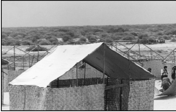
Shelters using BHR/OFDA-provided plastic sheeting are constructed to provide temporary housing for flood victims. (Photo by Alejandro James, BHR/OFDA/LAC)
