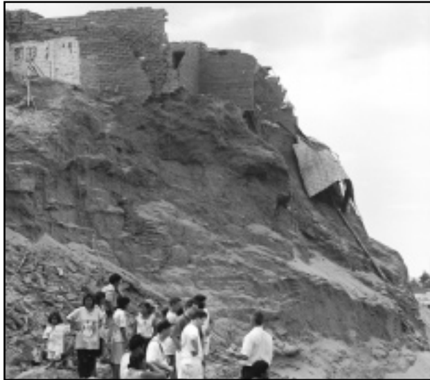
Houses built on a hillside in the village of Malpaso, Department of Trujillo, partially collapsed after heavy rains. (Photo by Alejandro James, BHR/OFDA/LAC)
