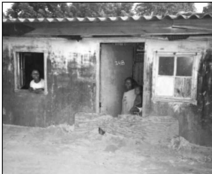
A piece of plywood protects the doorway of a residence in Kinshasa from sand left after floodwaters receded. (Photo by Regina Davis-Tooley, BHR/OFDA)
