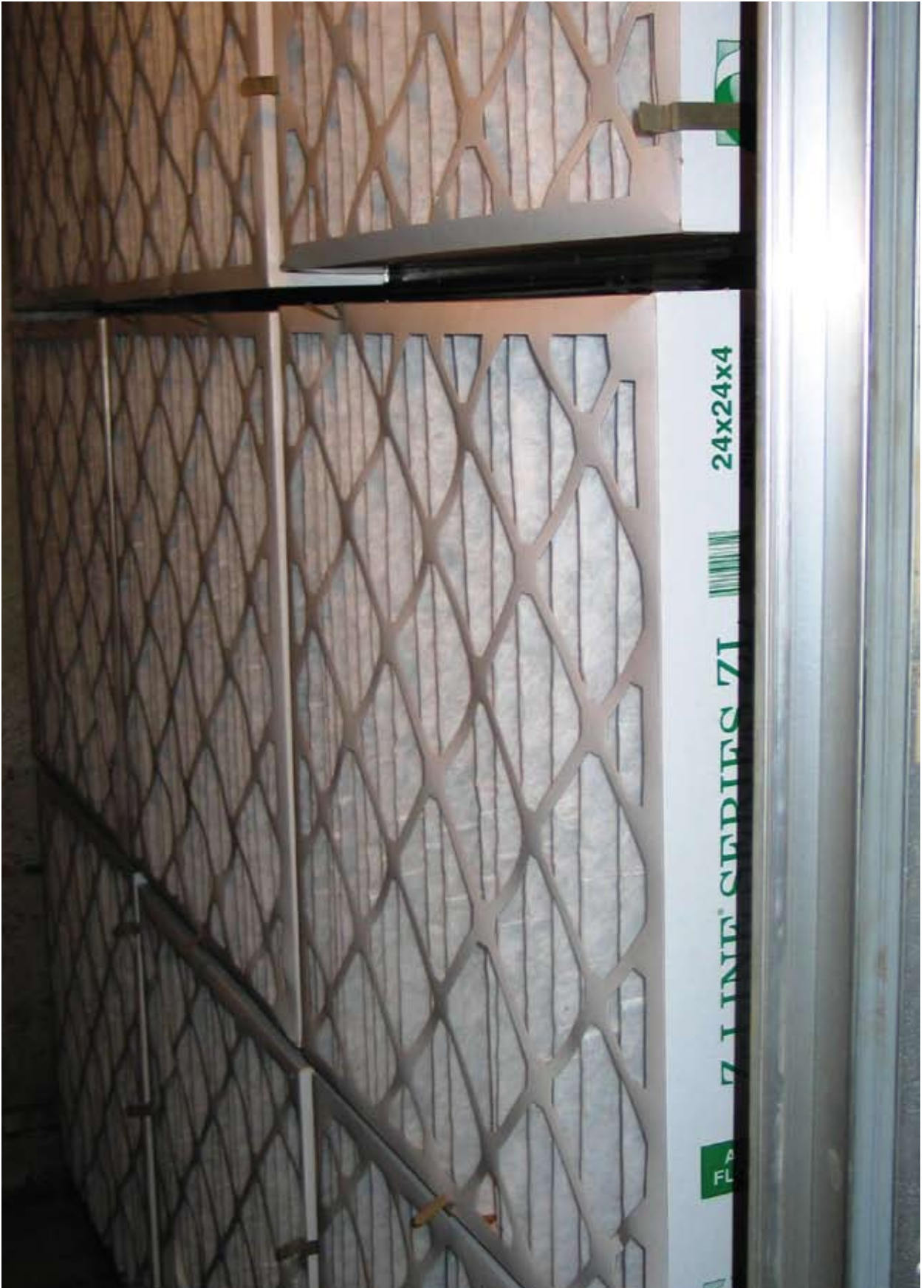
Figure C-6. Photograph of the 9-Filter Commercial HVAC System Used to Age Filters C14PCS and C11GM-16 (The test filters are behind the prefilters.)
