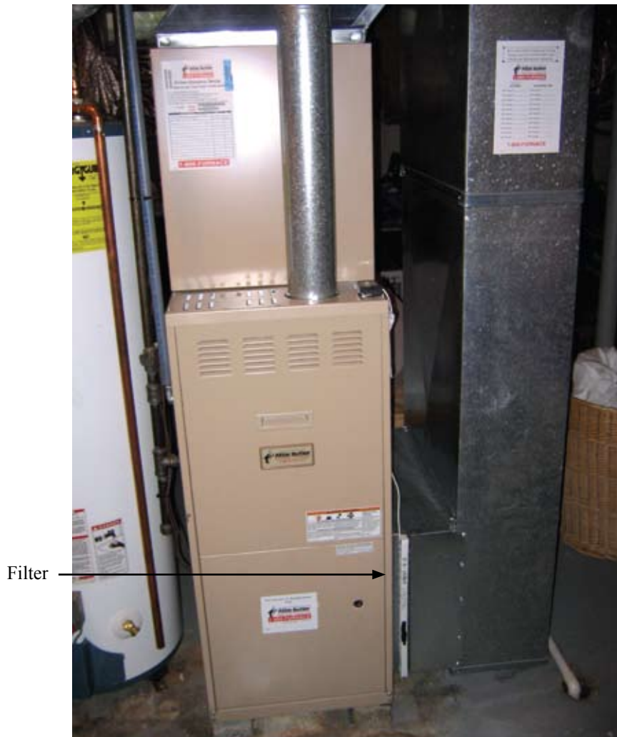
Figure C-1. Photograph of Residential HVAC System Used to Age Filter 6DDUE-8
