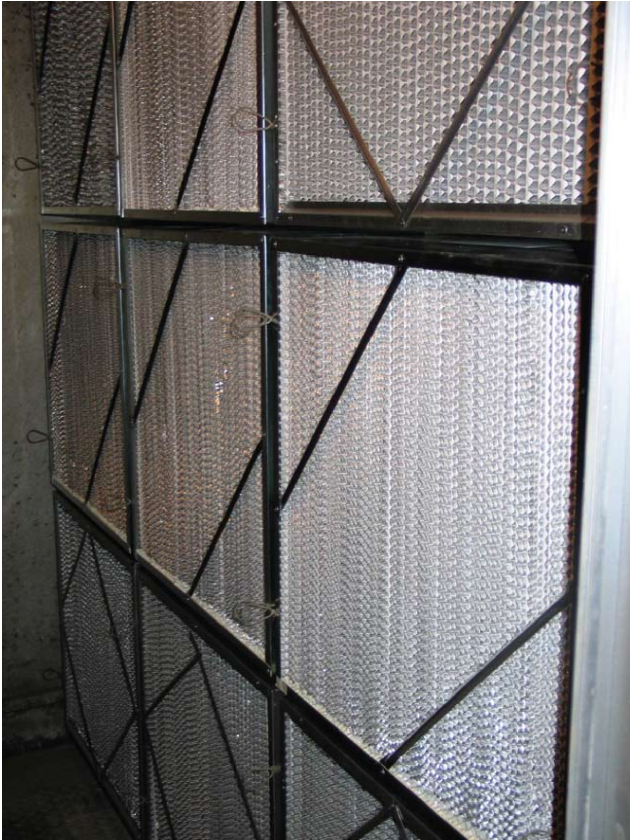
Figure C-5. Photograph of the 9-Filter Commercial HVAC System Used to Age Filters C14PCS and C11GM-16 (The test filters are shown before the prefilters were installed.)
