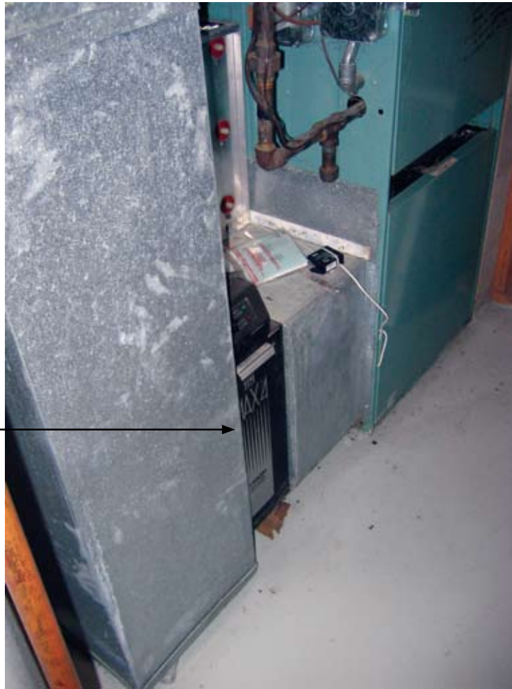
Figure C-2. Photograph of Residential HVAC System Used to Age Filter 8NM-10
