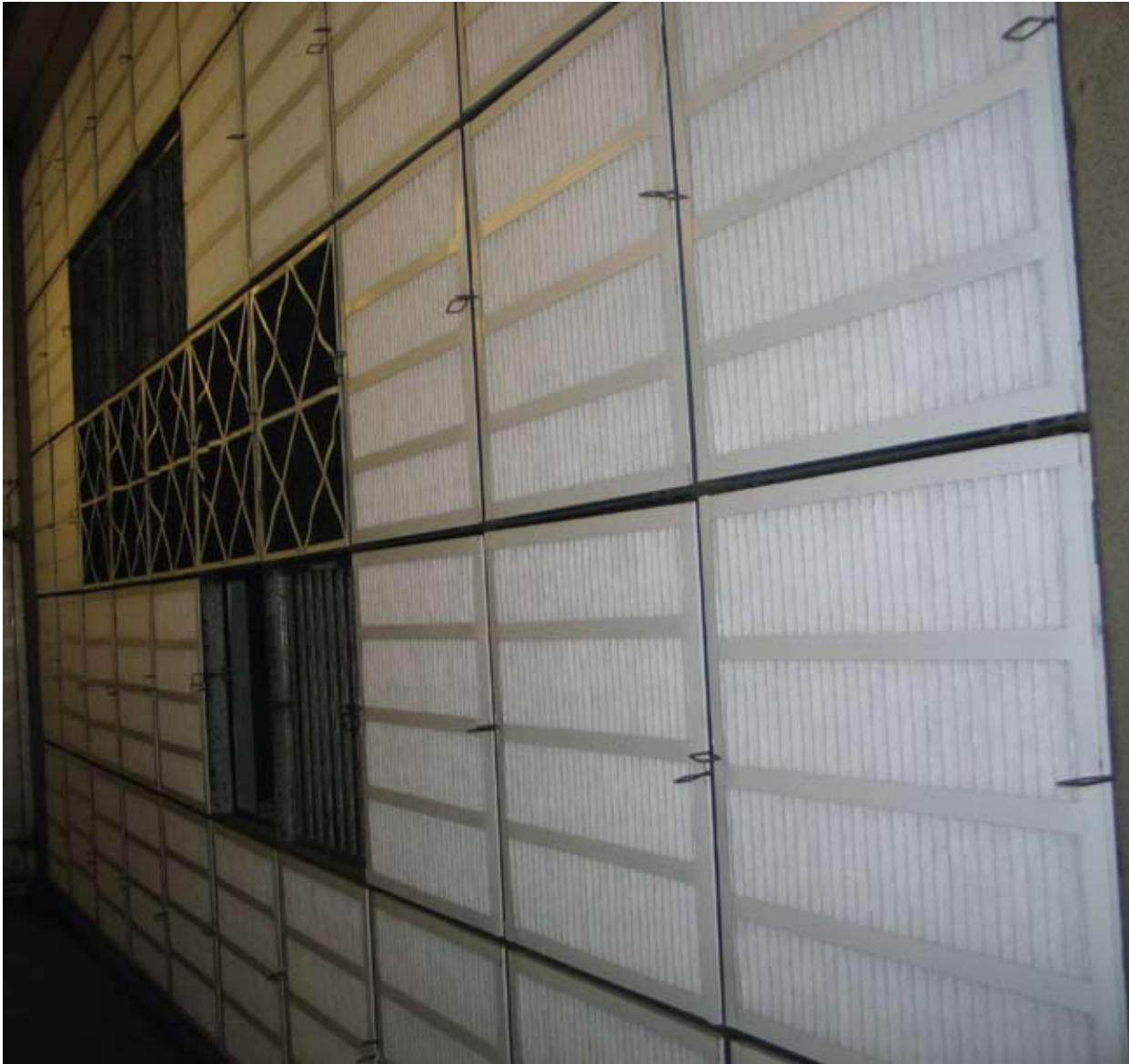
Figure C-3. Photograph of 40-Filter Commercial HVAC System Used to Age Filters C17FPP-8, C15AAA-11, and C8GZ-13 (C8GZ-13 Filters were inserted behind the prefilters in the gaps shown.)
