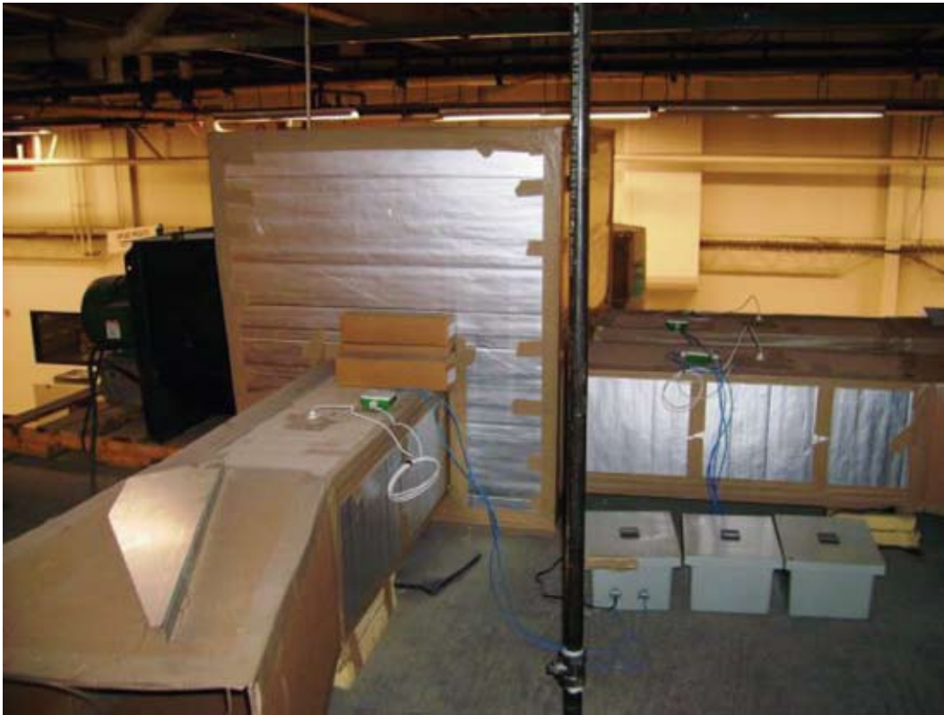
Figure D-8. Photograph of the Upstream Side of the Test Fixture and Airflow Controllers Used During the Ambient Aging of the Electronic Air Cleaners
