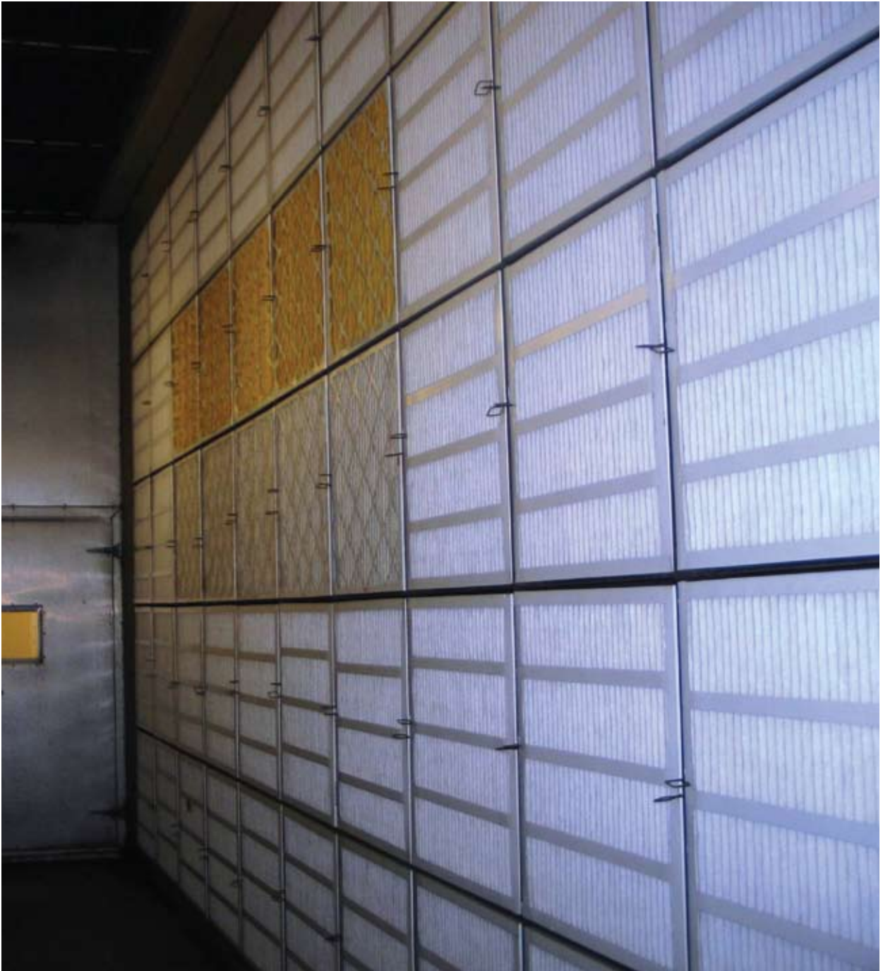
Figure C-4. Photograph of 40-Filter Commercial HVAC System Used to Age Filters C17FPP-8, C15AAA-11, and C8GZ-13 (The five C17FPP-8 and five C15AAA-11 filters are in the center.)
