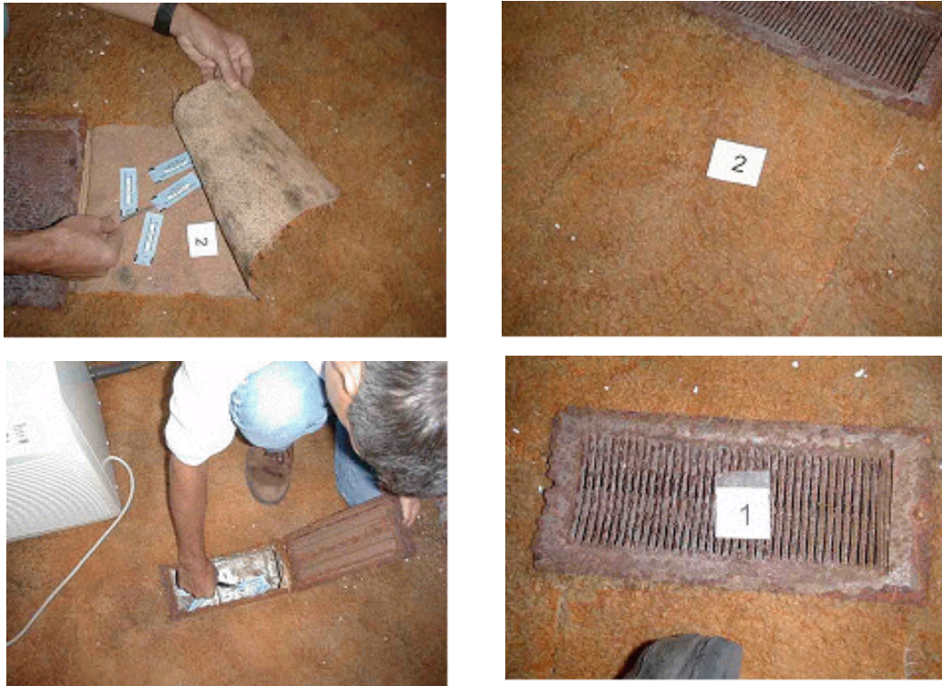
Figure 5.4-3. Spore strip sites 1 and 2 (see Table 1). Clockwise from top left: Strips in sub floor ducting under vent; vent in place. Strips under carpet; carpet in place.
