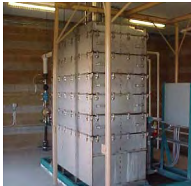
Air stripper treatment unit
