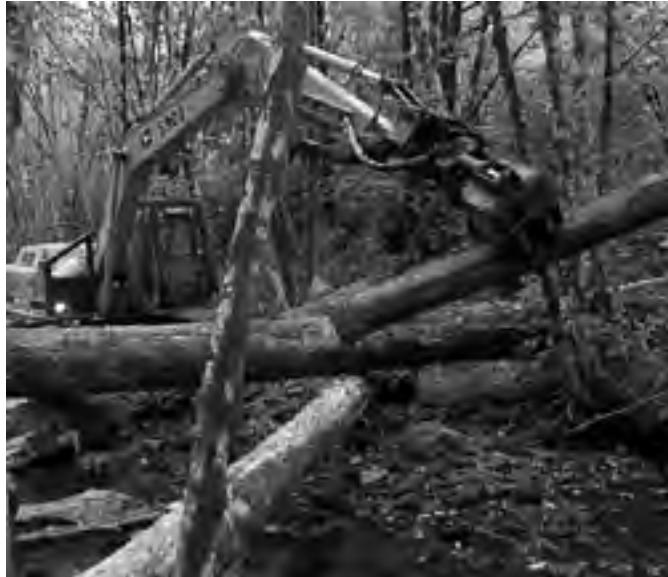
Figure 29. Alternative C would construct in-stream structures using heavy machinery and cabling as needed to assure stability.
