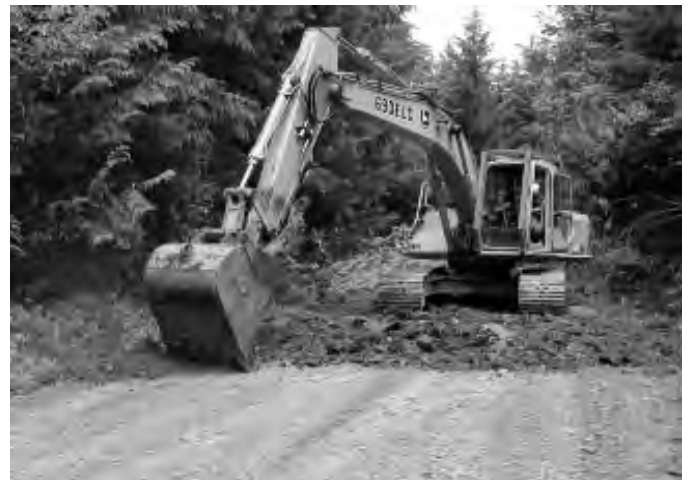
Figure 25. Extensive road decommissioning in Alternative B would reduce the establishment and spread of noxious weeds.
