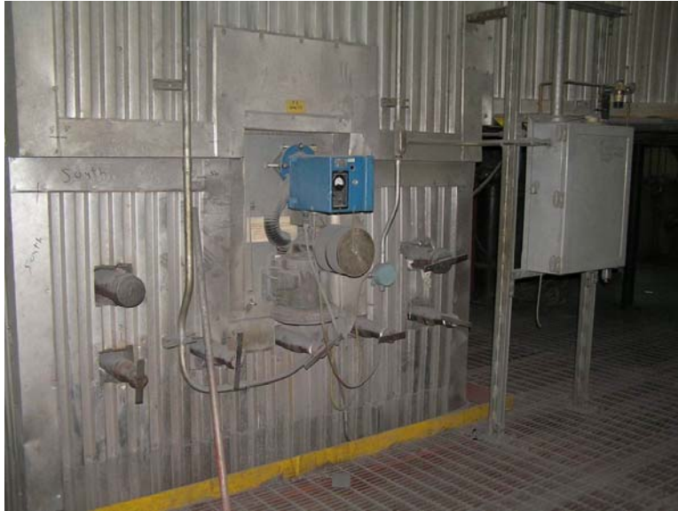
Figure 2-2. Emission Testing Ports for MP-5
