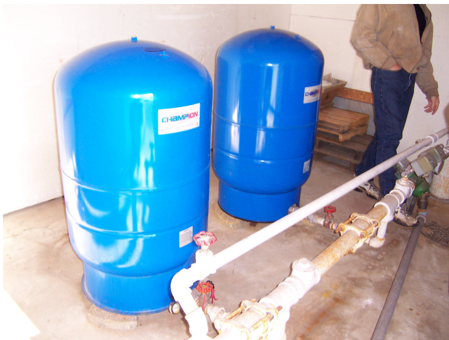
Figure 4-2. Existing Well Piping and Pressure Tanks at BSLMHP, MN Site
