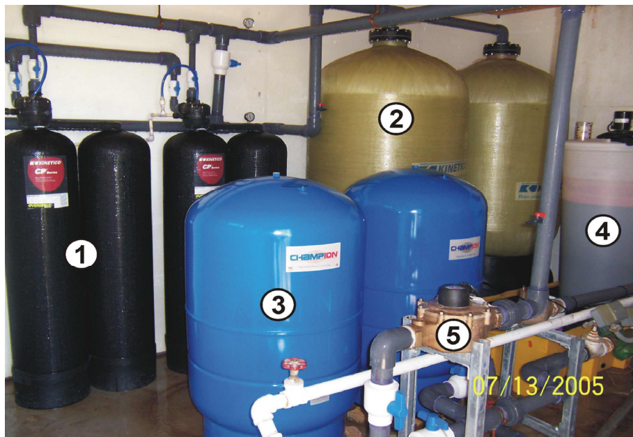
Figure 4-4. Photograph of Macrolite® Pressure Filtration System (1. Duplex Units, 2. Contact Tanks, 3. Pressure Filters, 4. Chemical Day Tank, and 5. Totalizer on Raw Water Line)
