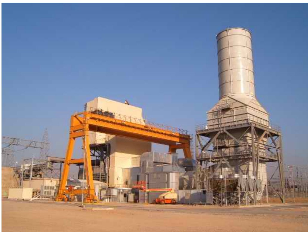
The fully operational V94 generator running at 260 MW. One of the largest and most efficient generators in Iraq, the V94 will help Iraqis face the approaching summer.
