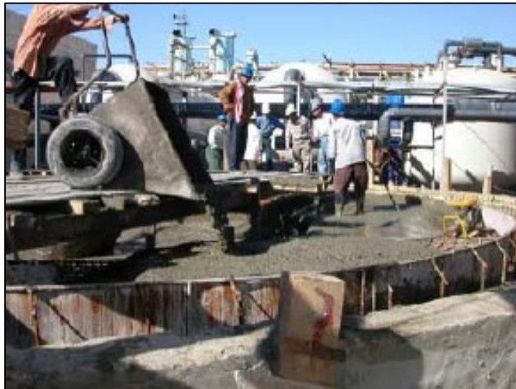
Workers lay a concrete foundation for water clarifiers at a power plant outside of Basrah. The water treatment facilities will improve efficiency and reliability of Basrah's power supply.
