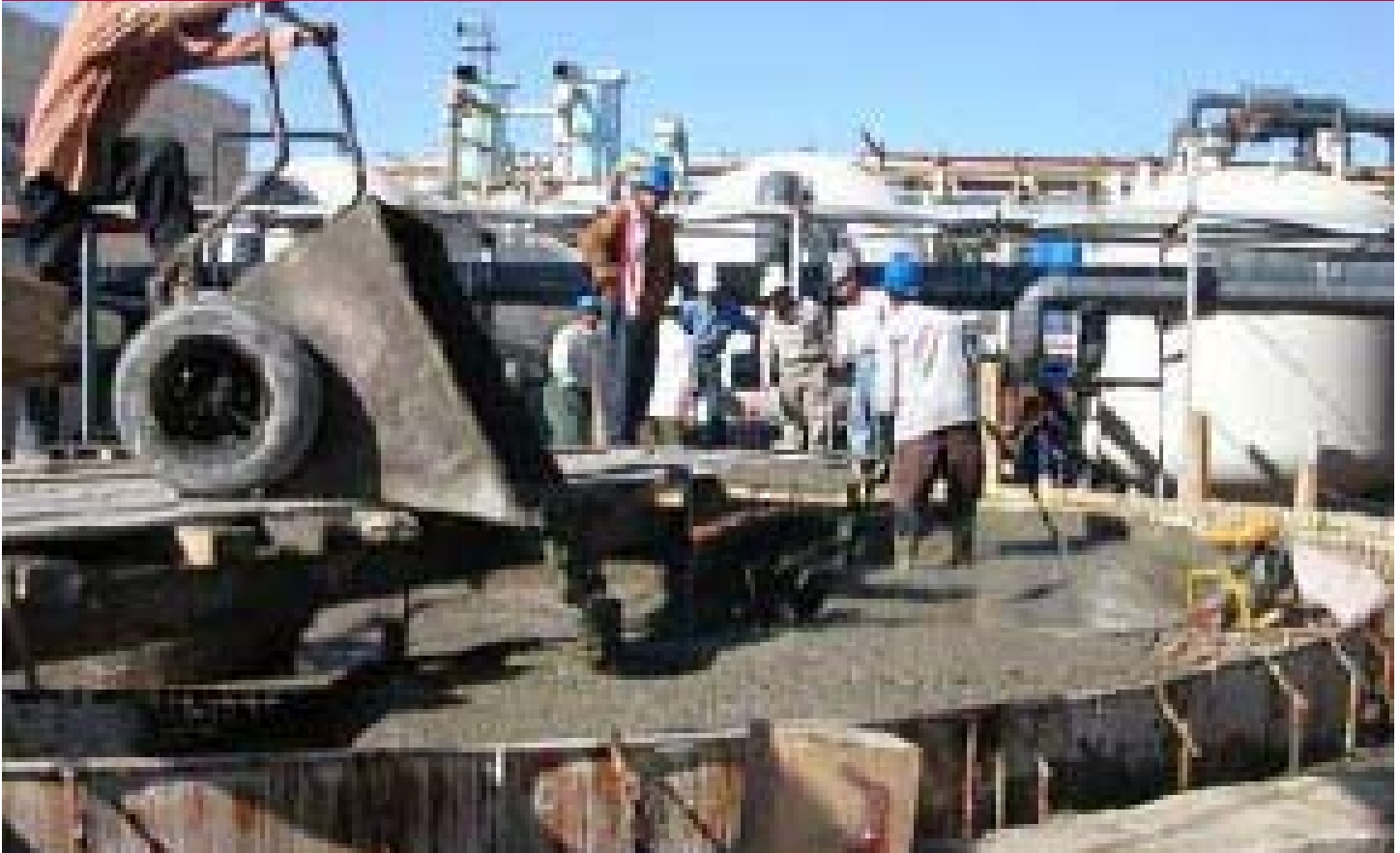
Workers lay a concrete foundation for water clarifiers at a power plant outside of Basrah.
