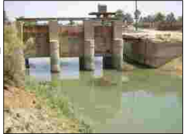
MOA/ARDI is repairing a water discharge regulator that will benefit over 7,000 Iraqis who live on the surrounding farmland.
