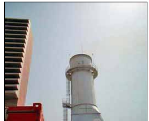
Expansion of the Baghdad south power plant is producing power to meet the summer demand peak. The project will add 212 MW to the national grid when finished in August.
