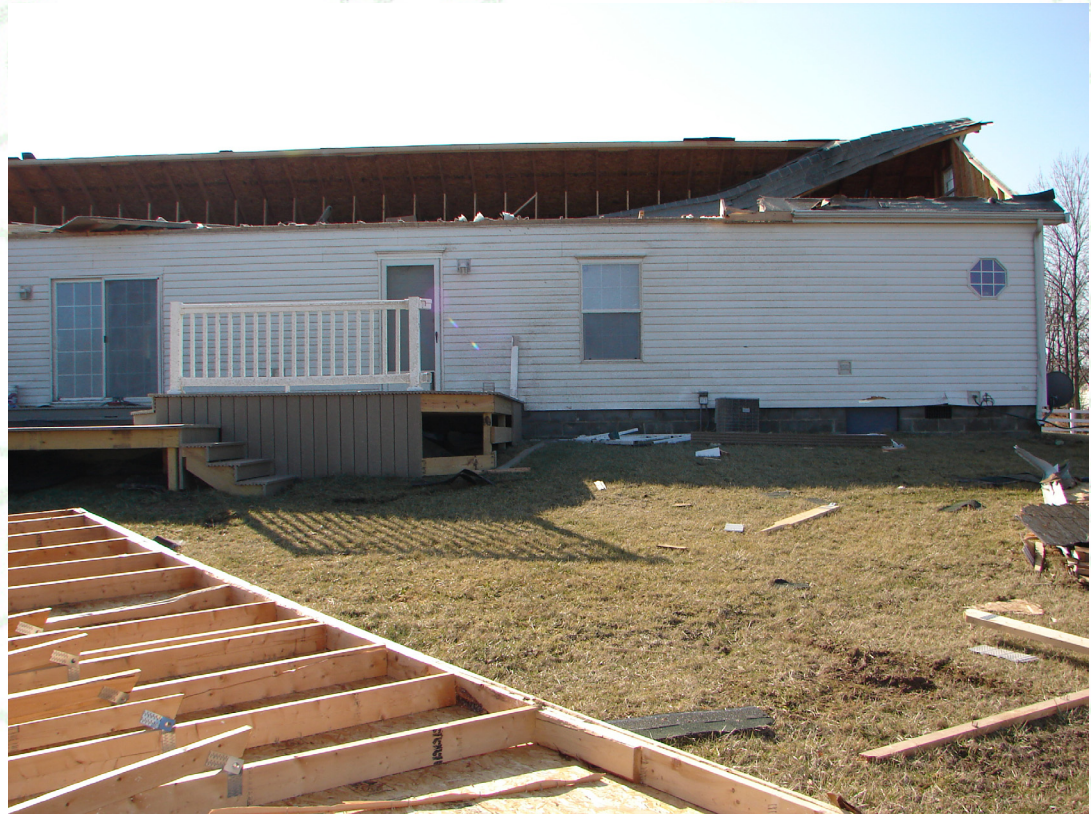
Above: An EF1 tornado touched down on February 11 near Muncie Indiana. The tornado had wind speeds of nearly 100 mph as it damaged this home.
