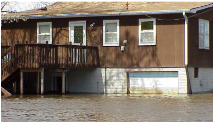
This house was properly elevated. Some time after the permit was issued, the owner improved the lower area and subsequently suffered flood damage. This shows the benefit of requiring lower areas to stay open.
