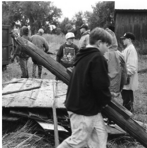
Boy Scouts cleared debris to improve wildlife habitat at Altman Confluence Tract, Montana.
