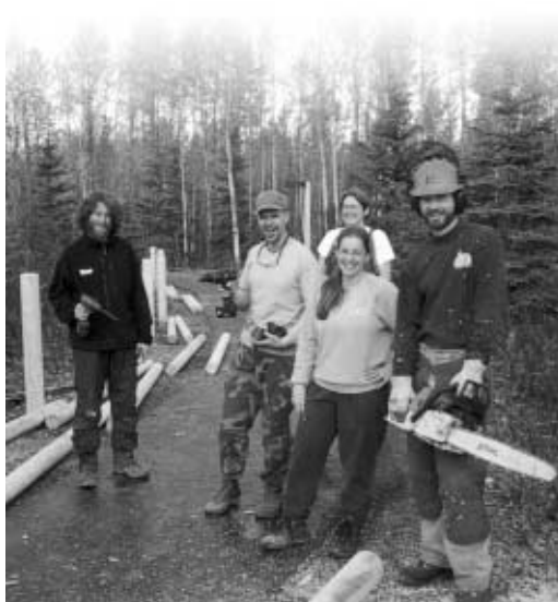
Although plans for National Public Lands Day included having work crews install only support posts for a fence near the Campbell Creek Science Center, enthusiastic volunteers got the entire fence built.
