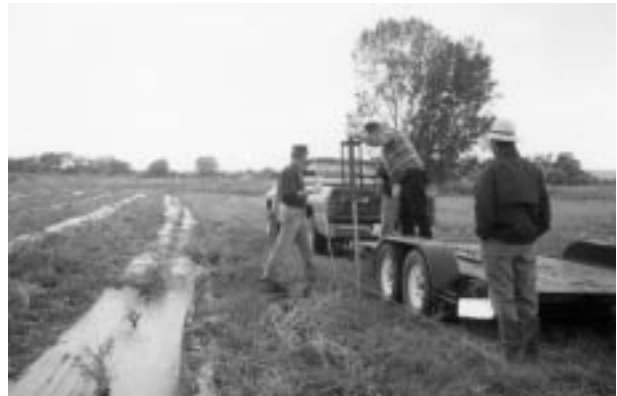
National Public Lands Day volunteers helped to construct a shelterbelt electric fence to protect young trees and shrubs at Montana's Altman Confluence site.
