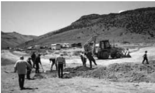
The Cache Peak Back Country Horsemen constructed a turn-around loop with pull-outs at the Big Cottonwood Creek Trailhead in Idaho, saving BLM about $10,000 in contracting expenses.
