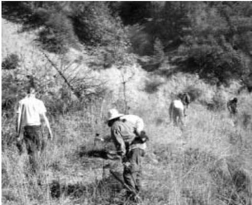
Construction of 1.5 miles of the Grayback Mountain Trail was one of two National Public Lands Day projects in the Medford District. When complete, this trail will link with the Pacific Crest and Boundary trails, providing access to more than 2,500 miles of trail in the western United States.
