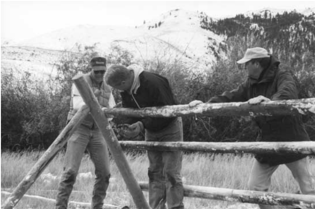
Montana State Director Mat Millenbach (in white hat) and Dillon Field Manager Scott Powers assisted a volunteer in constructing jack-leg fencing around the homestead cabin at the Beaverhead River site on National Public Lands Day.
