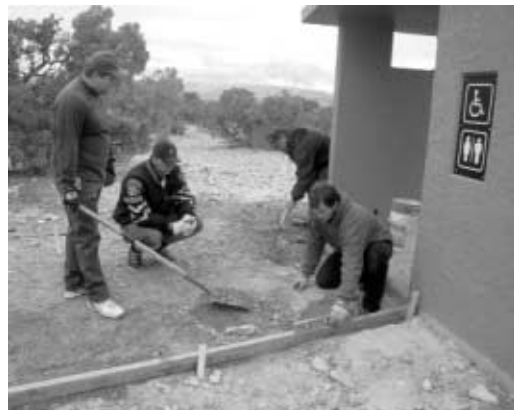
National Public Lands Day volunteers in Utah engaged in many projects at the Wedge Overlook near Price, including pouring concrete for a ramp to make the vault toilet accessible to persons with disabilities .
