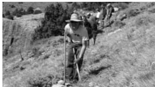
Volunteers constructed one-third of a mile of trail at the Sinks Canyon climbing area, just west of Lander, Wyoming.
