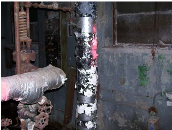
Crumbling asbestos-containing insulation on pipes.
