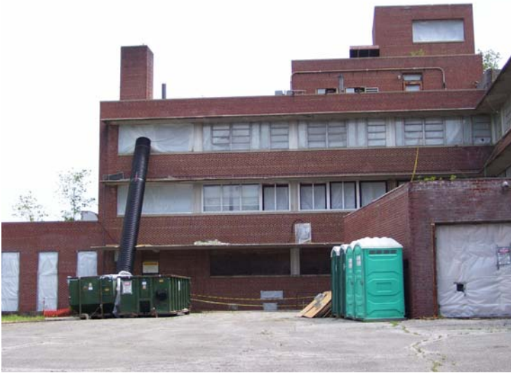
To enable safe asbestos removal, (sometimes broken) window glass was removed and the building was sealed.
