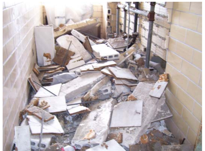
Debris containing haz mat, medicines and old paperwork.
