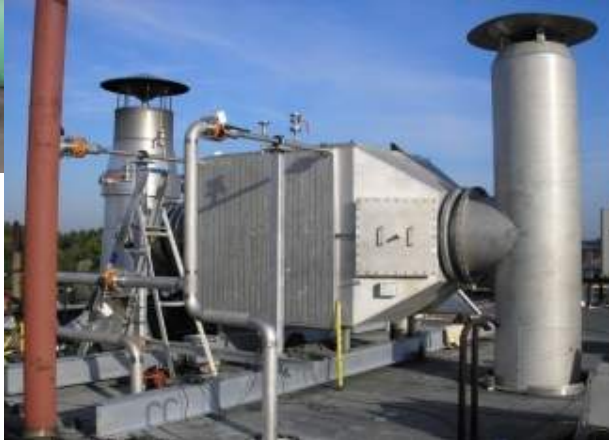
Janssen Beerse, Belgium Stack Gas Economizer
