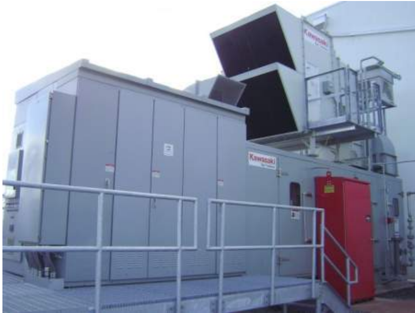
OCD – Raritan, NJ Gas Turbine
