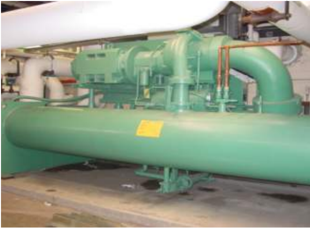
Ethicon Somerville, NJ Upgraded Chiller with VFD
