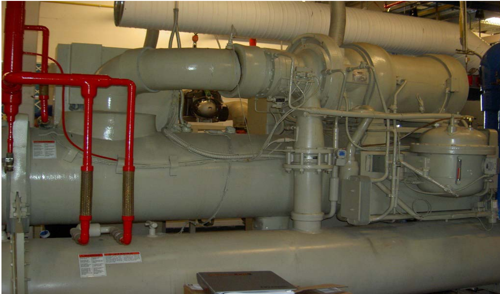
A 250 Ton Centrifugal Chiller Before
