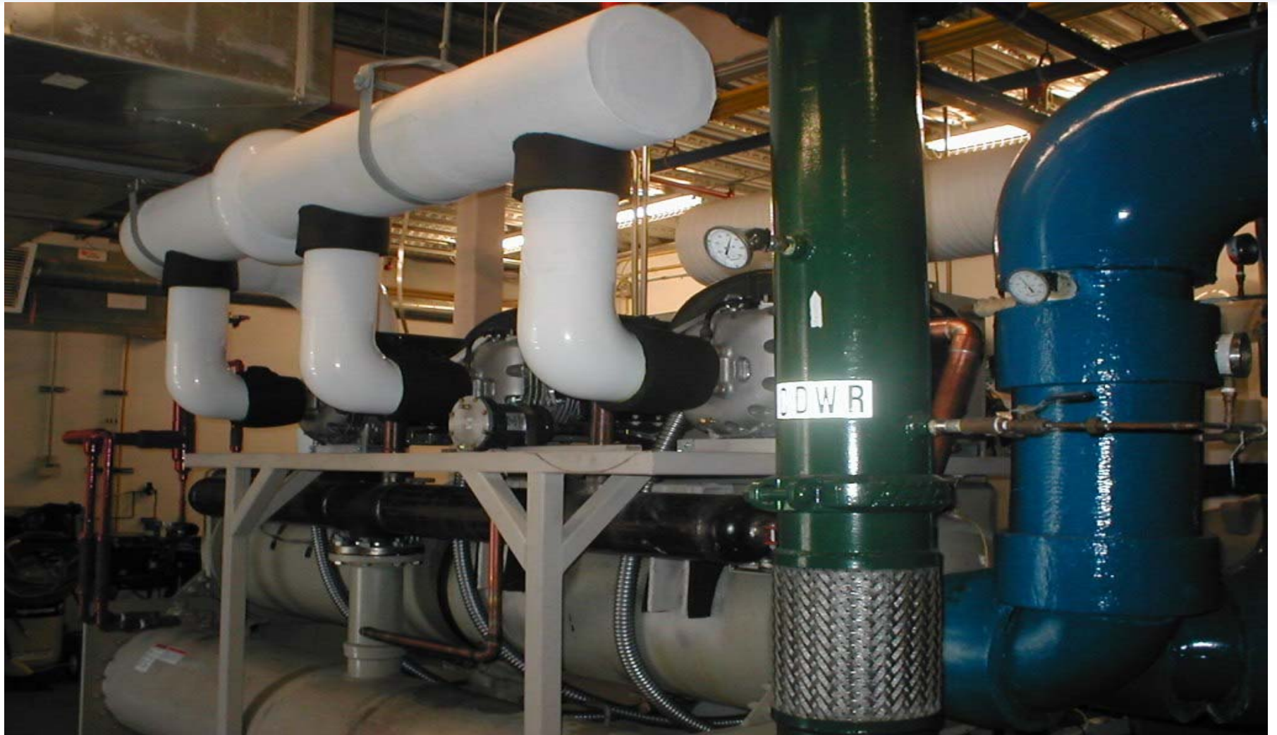
A 250 Ton Centrifugal Chiller After
