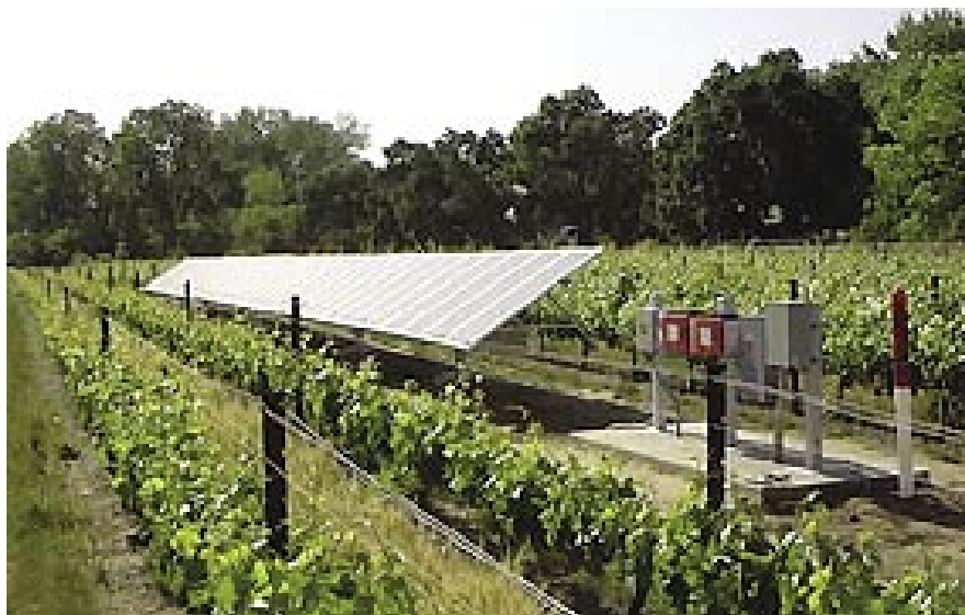
Renewable Technologies, Inc. installed this 5-kW, ground-mounted PV system at Bokish Vineyard in California's Central Valley. (Photo by Renewable Technologies, Inc.)
