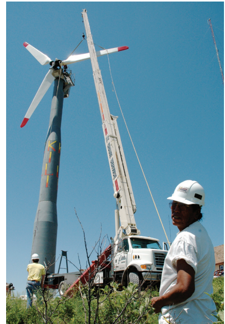
A crane places blades atop the KILI wind turbine. The station will use the electricity and sell the excess generation to its utility, LaCreek Rural Electric Cooperative. (Photo by Intertribal Council on Utility Policy)
