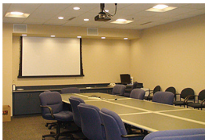
By replacing all the conventional lights with 12-watt LEDs, Tri-State reduced energy consumption in its two conference rooms by more than half when all the lights were in use. (Photo by Tri-State Generation and Transmission Association)
