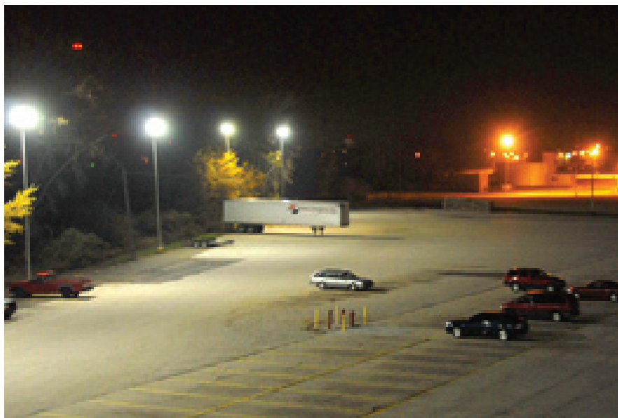
A parking lot lighting project in Manitowoc, Wis., replaced the four lamps in the foreground with fluorescent units that operate at 234 watts. Compare the upgraded lights to the HID legacy lamps in the background that operate at 1160 watts. (Photo by Orion Energy Systems)
