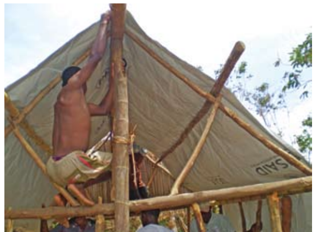
Following Cyclone Ivan, residents of Madagascar construct a new roof with plastic sheeting from OFDA (Courtesy of CARE).
