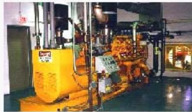
Internal Combustion Engine (range from 100 kW to 3 MW)
