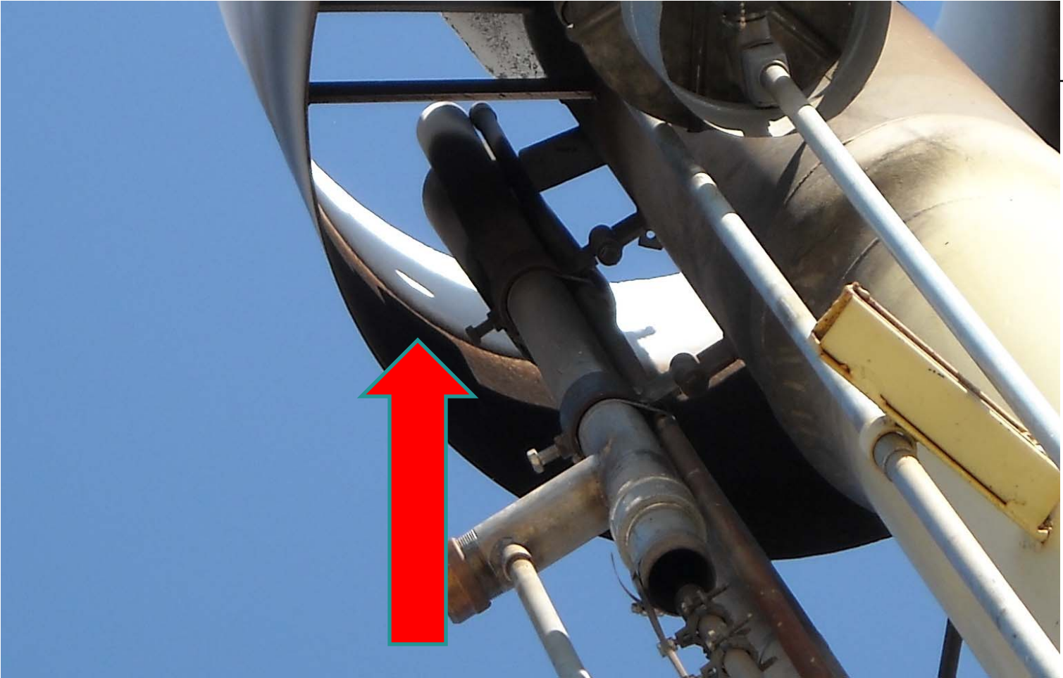
SILICA BUILD UP INSIDE THE FLARE HOUSING
