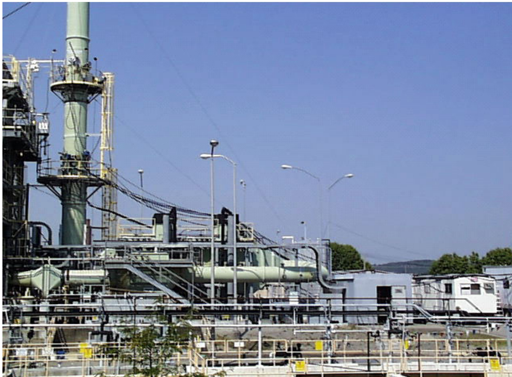
Figure 3-3. Side View of TSCAI Stack. Sampling platforms are at the left and CEM trailers are at the lower right.
