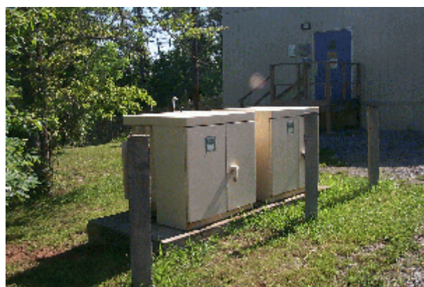
Figure 5-4. Transformers at ORNL containing oils with PCB concentrations greater than 50 ppm.
