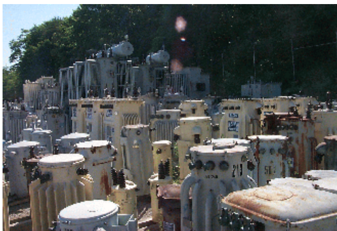
Figure 5-3. Transformer yard at ORNL.
